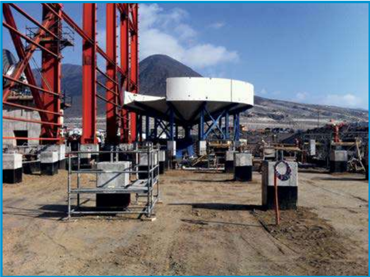
Hidroseparator, Planta Pellets, Huasco - Chile
